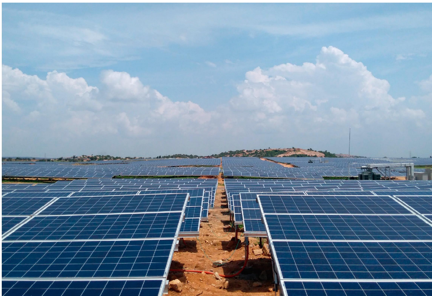
This 100 MW solar park in Telangana, India, was developed by Adani and utilizes string inverters from Huawei.
