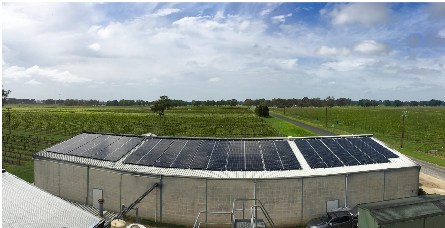
Solgen developed this 100 kW solar system on the rooftop of Hollick Wines winery and restaurant in Coonawarra, South Australia. The project is estimated to have reduced the winery's consumption of on-grid electricity by more than 50%.
