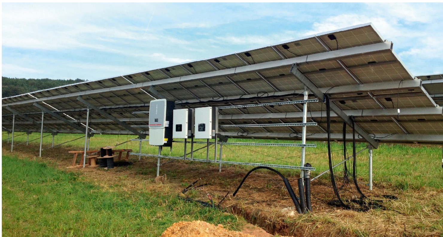
Huawei inverters installed at a project in Parsberg, Germany. Germany's Renewable Energy Sources Act, promulgated in the year 2000, provided the foundations for the energy transition. China is also undergoing its own massive energy transition with huge amounts of new PV being connected each year.
